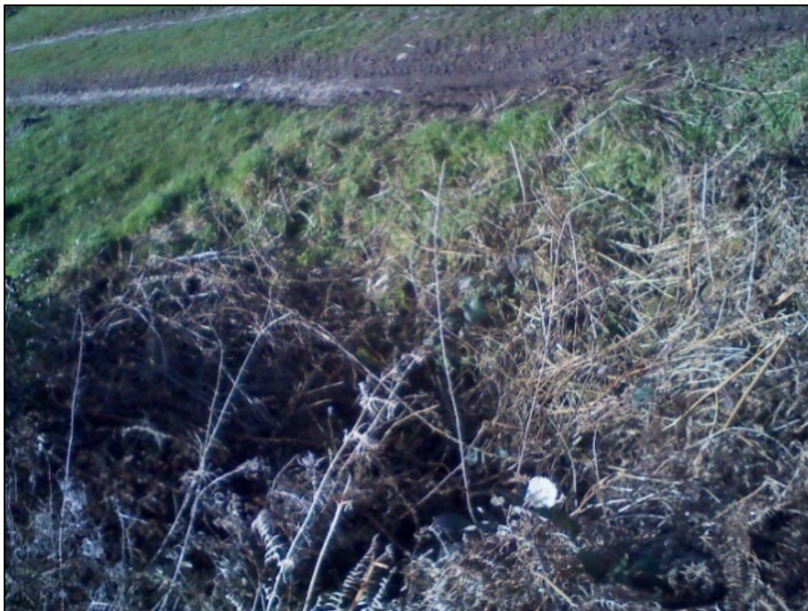
Figure 3-4 Field culvert structure TT01_0507 – TT01_0500 (Downstream face, obscured by vegetation)
